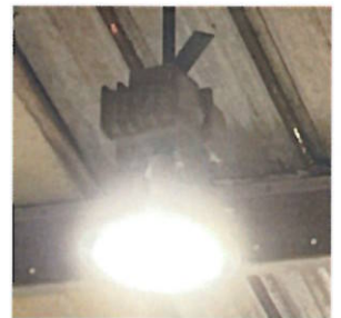
New LED Lighting
